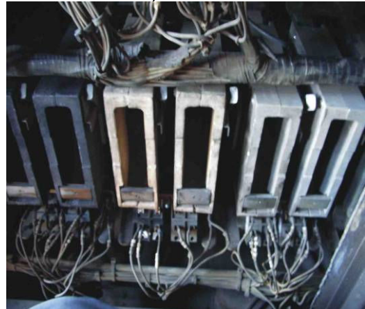
Engine room arc chute in an X class The black coloured arc chutes to the left were found to contain bonded asbestos.
