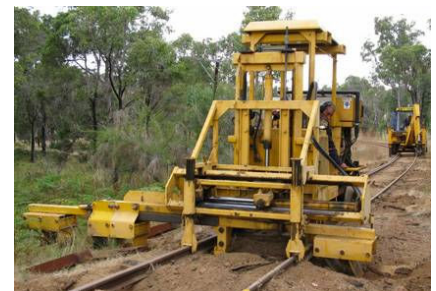
A big job calls for the right equipment - a linear scarifier at work on the Hotham Valley line.
